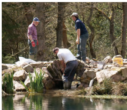
Philip Dolphin ( centre ) using traditional techniques to build the arched dry stone bridge, assisted by Mick Saunders ( left ) and Andy Carr ( right ) ( Photo: Anne Tupholme )
